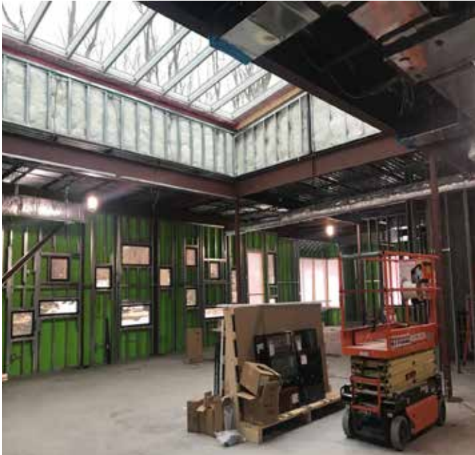
Interior walls and windows are being installed on our 6,555 square foot childrens addition at the east end
